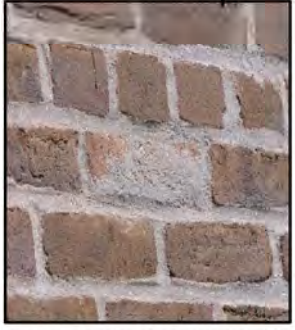
Over pointed repair in 1979
