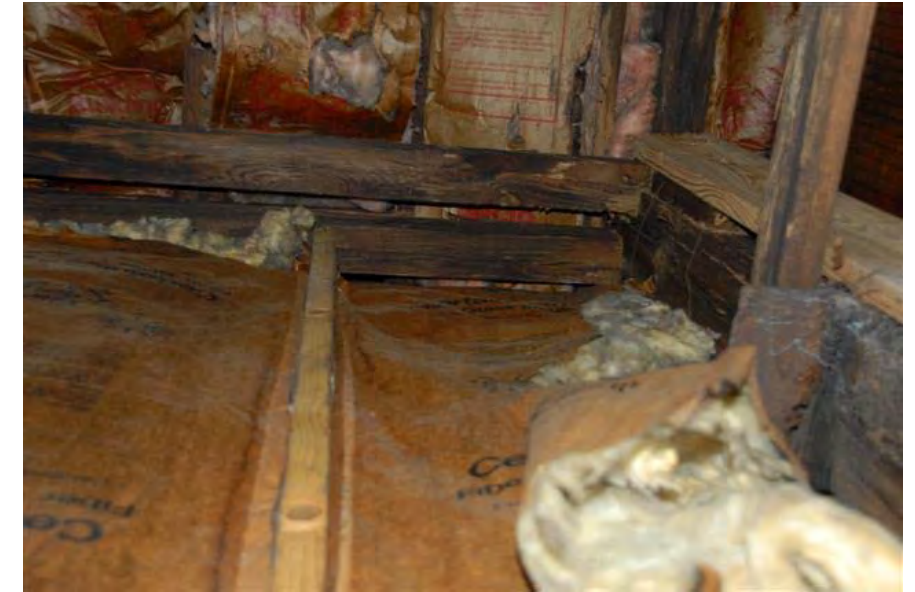
Double Beam across the gable wall, original post shows signs of deterioration; new board material attached to support the horizontal load (southeast corner).
