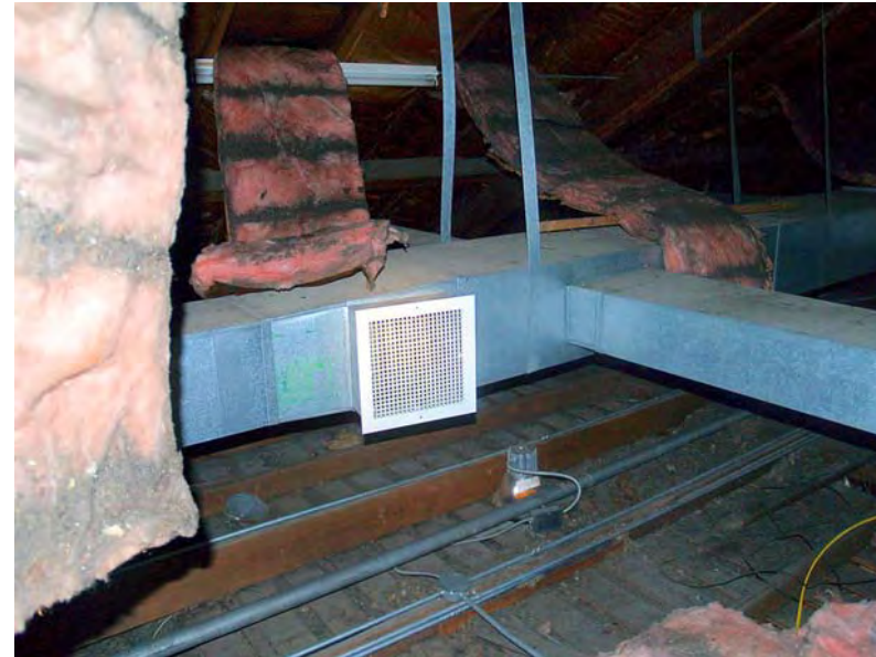
3- Supply Grille Discharging Into Attic
