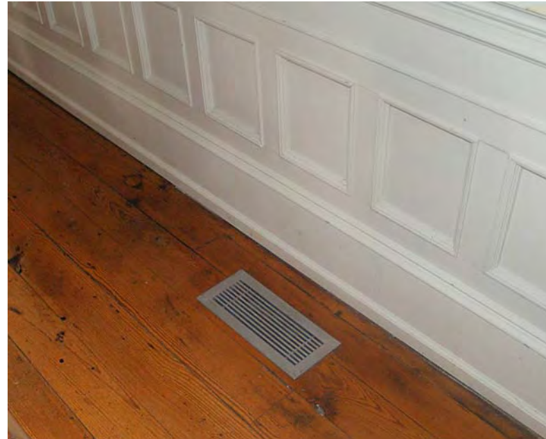
14 Floor Register for Heating
