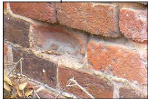
Eroded brick in lime mortar not repointed in 1979
