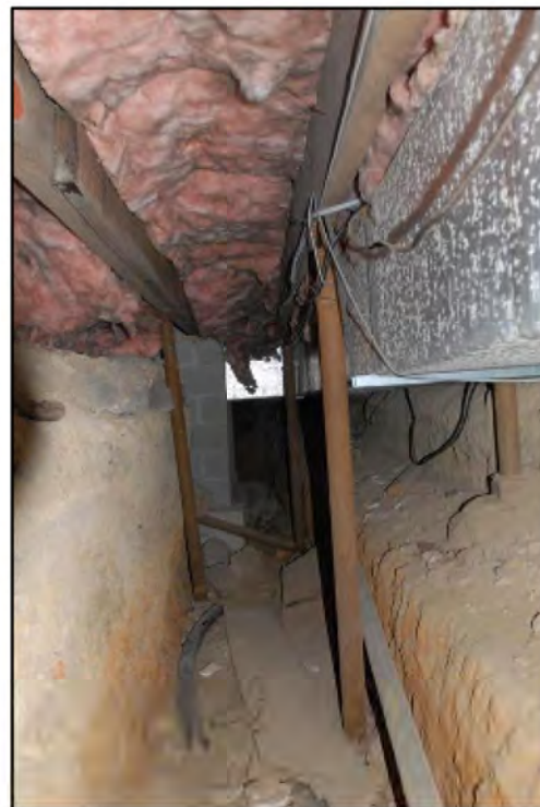
Granite exterior foundation wall to the left, ductwork on compressed soil to the right
