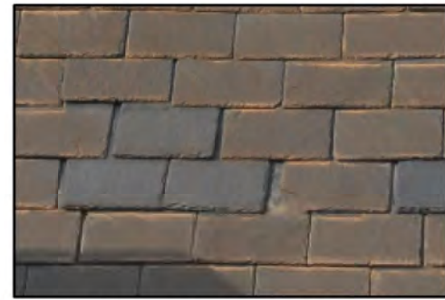
Black replacement slate is not wide enough
