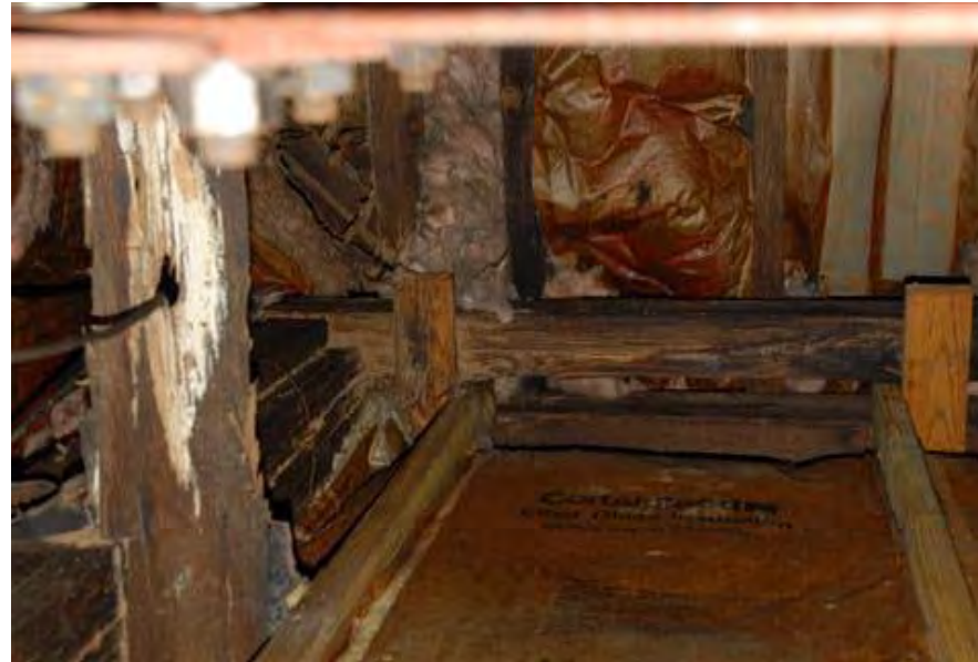
Double Beam across the gable wall and original post all shows signs of deterioration; (southwest corner).
