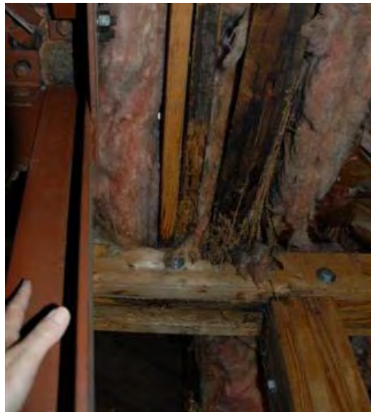
Floor joists for belfry floor, outside of the steel frame, SW corner
