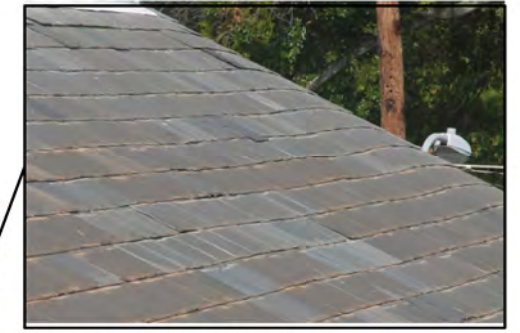
Sagging eave (curved surface)
