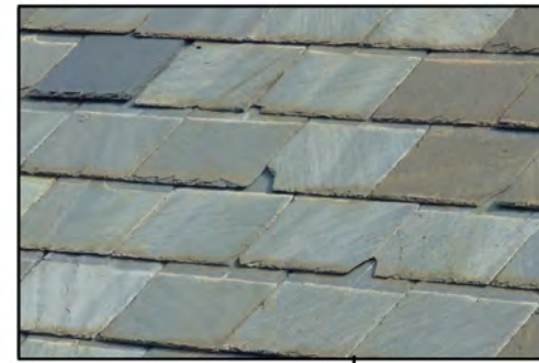
Chipped corners of original slate
