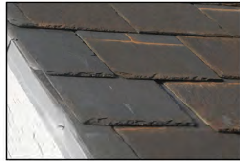
Black replacement slate does not match size of previous tile
