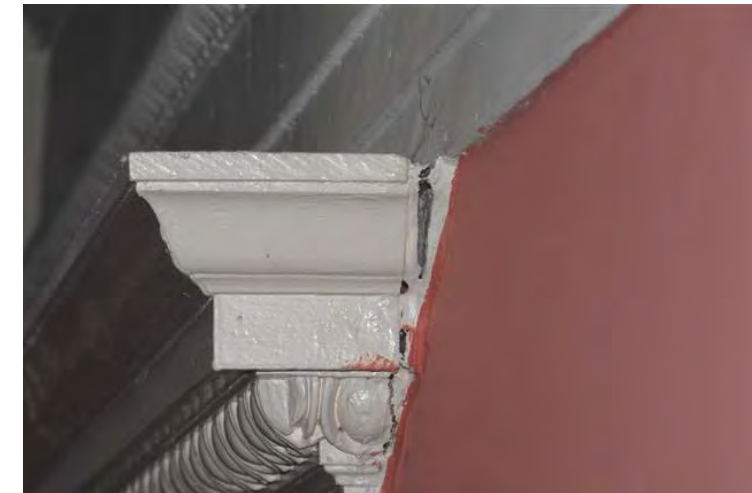
Window 4: Header trim detaching
