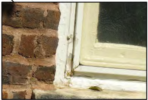
Stress crack in masonry next to granite sill
