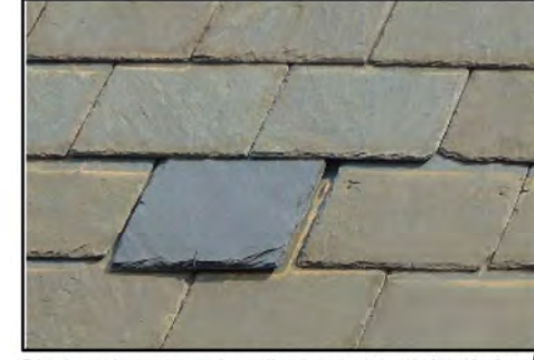
Black replacement slate tile does not match existing
