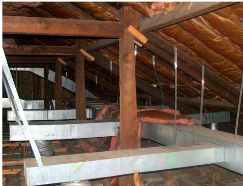
4- Internally Insulated Duct in Attic
