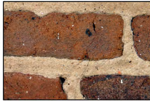
Strongly weakened masonry- cracked brick and mortar
