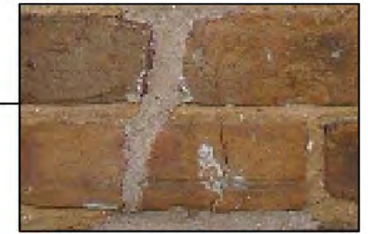
Cracked brick and non-matching mortar (1979)
