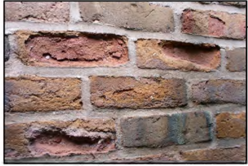
Spalled/ eroded brick with 1979 mortar
