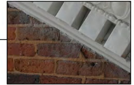
Oversprayed white paint on brick
