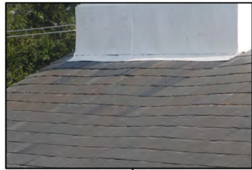
Sagging eave roof plane
