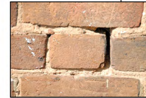
Failing lime mortar
