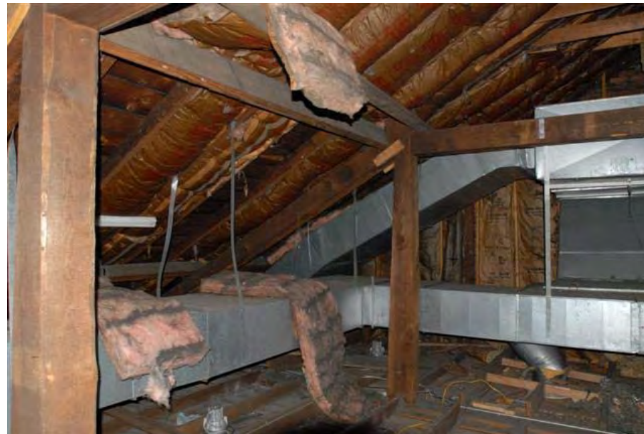
Original 1853 heavy timber framing in the attic; note insulation detaching from roof underside.
