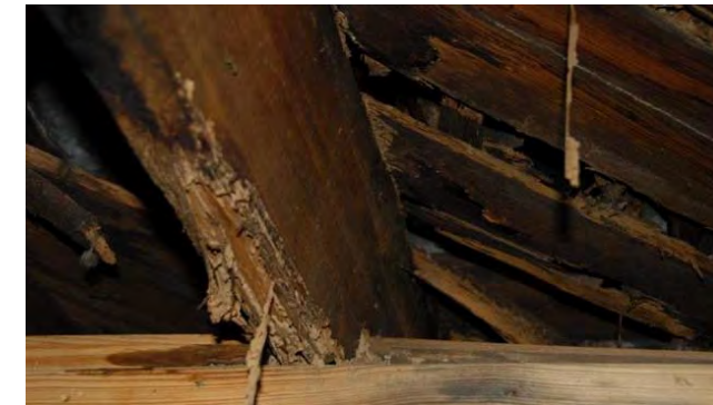
Water damage to beam at belfry floor, NW Corner
