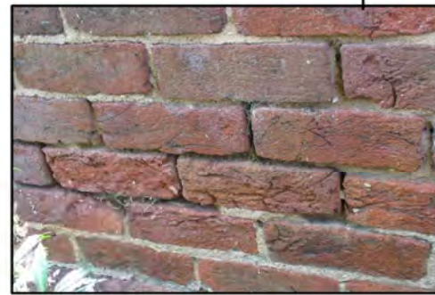
Eroded brick, failing lime mortar not repointed in 1979
