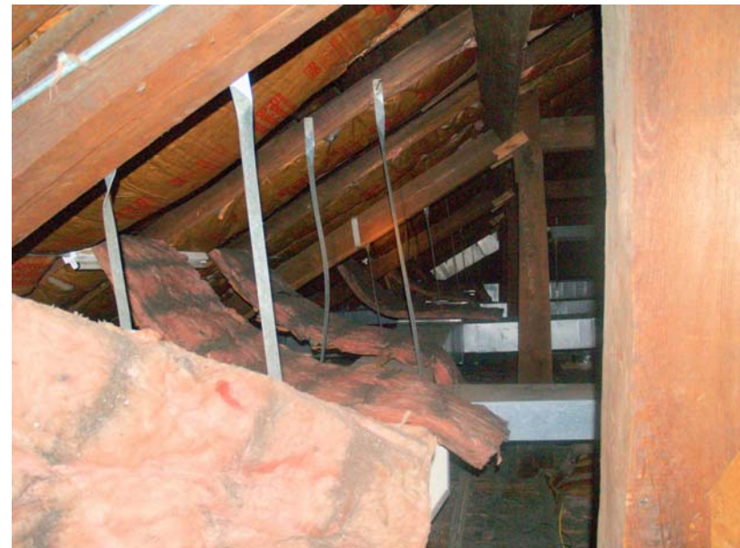
2- Fallen Roof Insulation in Attic
