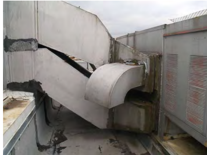
7 Outside Air Intake for Rooftop Unit
