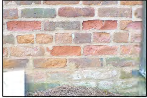
Spalled/ eroded brick
