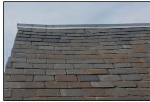
Sagging ridge line with black replacement slate tiles
