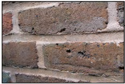
Failing brick surfaces
