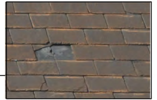
Missing slate tile
