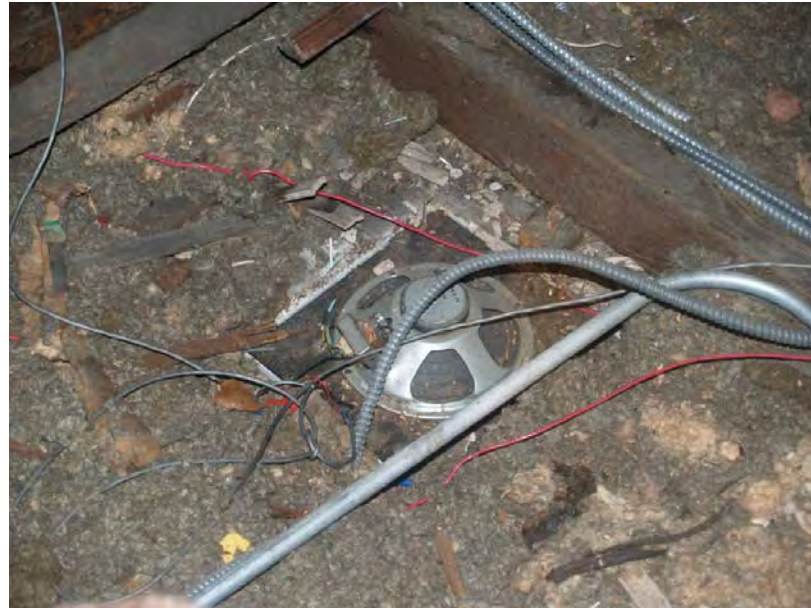
Speaker in Ceiling (from Attic)
