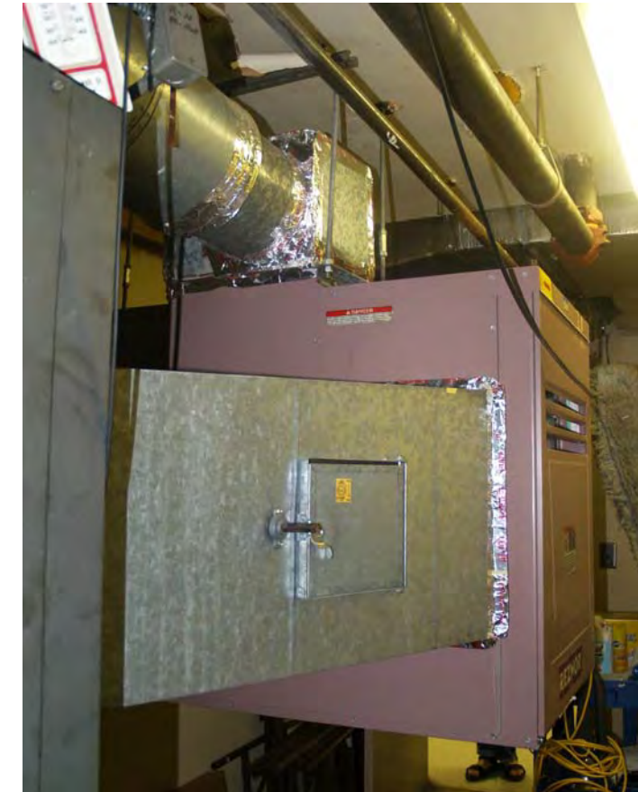
11 Gas Fired Heater for Sanctuary
