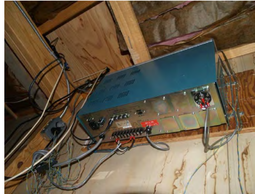
Amplifier in Organ Blower Room
