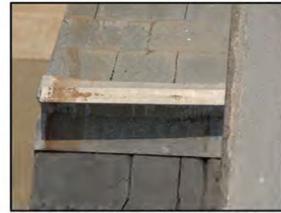
Corroded gable cap on slate roof exterior of gable wall
