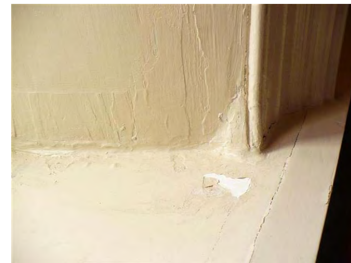
Window sill with old paint layers and new peeling
