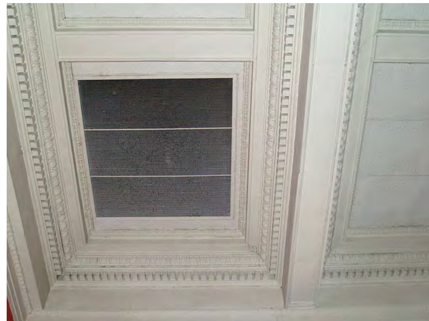
13 Return Air Grilles for Sanctuary Cooling
