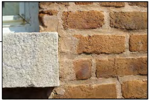
Over use of repointed 1979 mortar next to sandblasted granite sill
