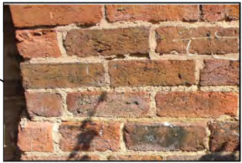
Eroded brick with deteriorated mortar
