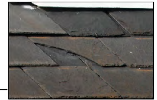
Major chip in slate tile
