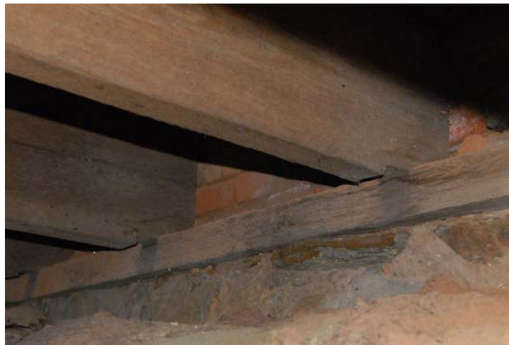
Floor joists on top of the granite foundation wall, at the base of the exterior brick wall.
