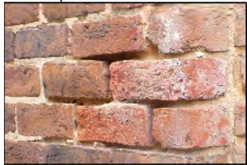
Eroded/ spalled brick with eroded lime mortar
