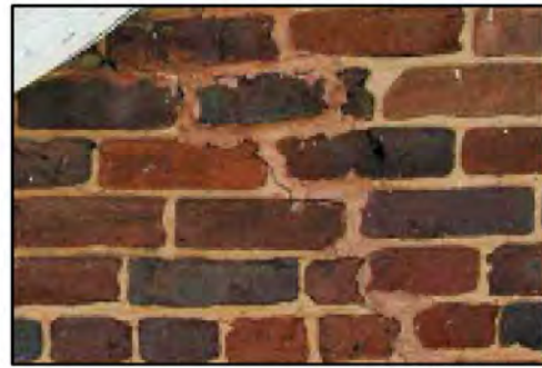
Poorly repaired masonry crack (1979)
