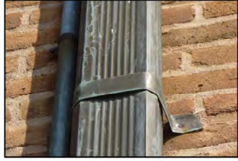
Rusting nail fastened into brick
