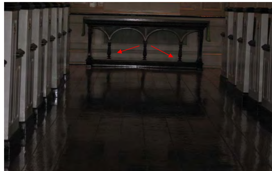
Photo 2 – Slab depression at sanctuary floor
