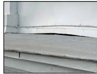
East side flashing gap, built-up roofing
