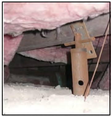
Steel post failing to support joist
