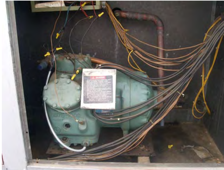
9 Rooftop Unit Compressor-Good Condition
