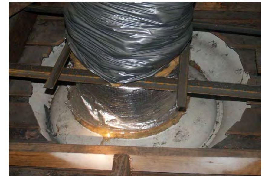
6 Un-Insulated Diffuser back in Attic-Needs to be Insulated
