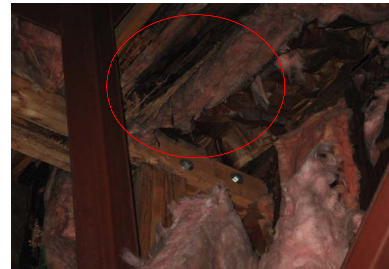
Photo 16 – Damaged Wood below Steeple
