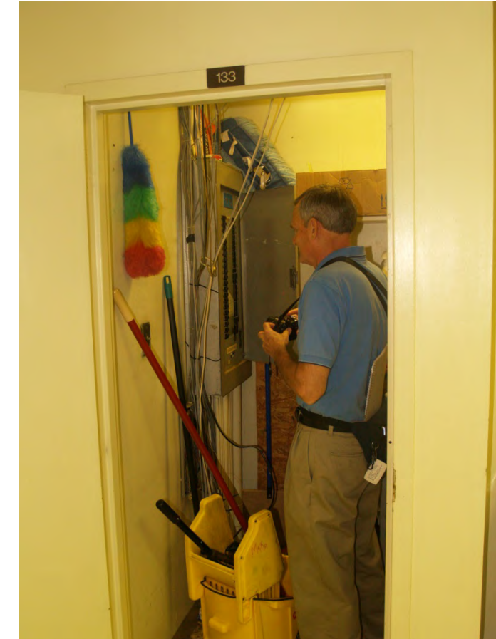
Electrical Panel Serving Sanctuary
