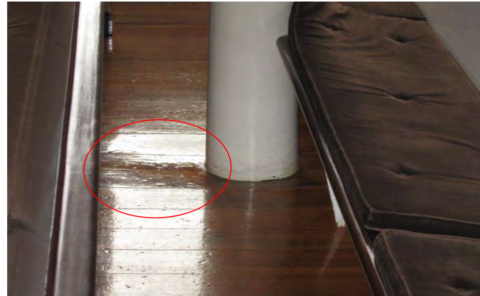
Photo 1 – Slab depression at Post Base
