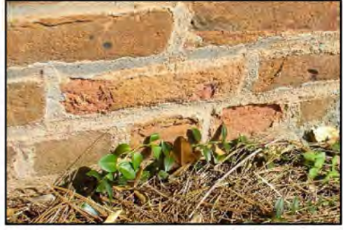
Spalled brick with repointed 1979 mortar
