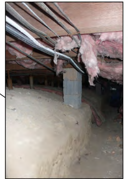
Concrete block supports too close to edge of compacted soil
