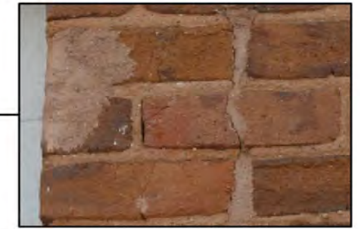
Over pointed mortar (1979)
