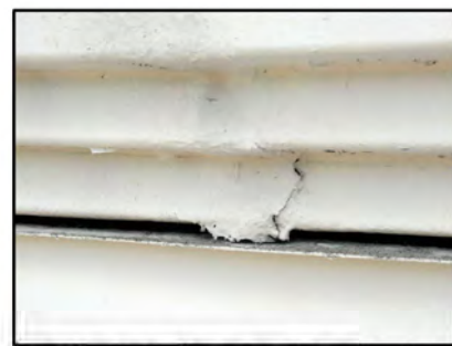
Cornice and frieze- not weathertight
