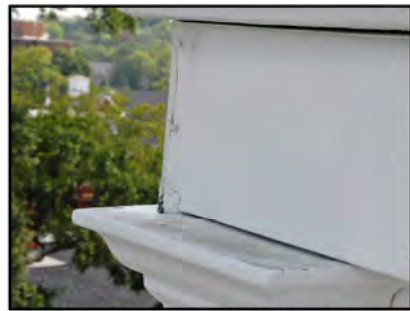
Capital detail- not weathertight
