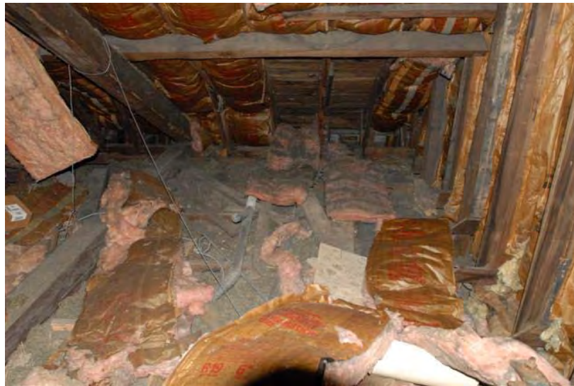
Failing insulation in the front section of the attic
