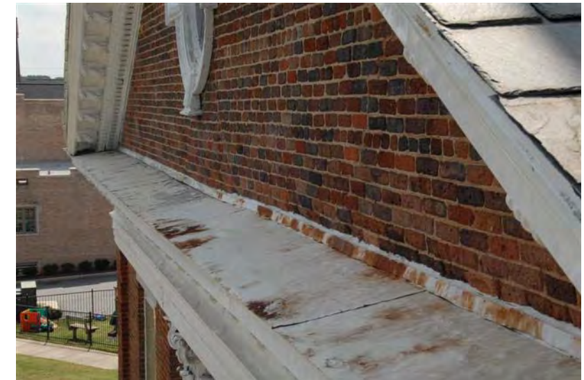
Cover metal sheet across the horizontal cornice at east gable
