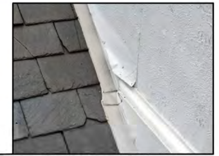
Flashing detail- metal skin not weathertight
