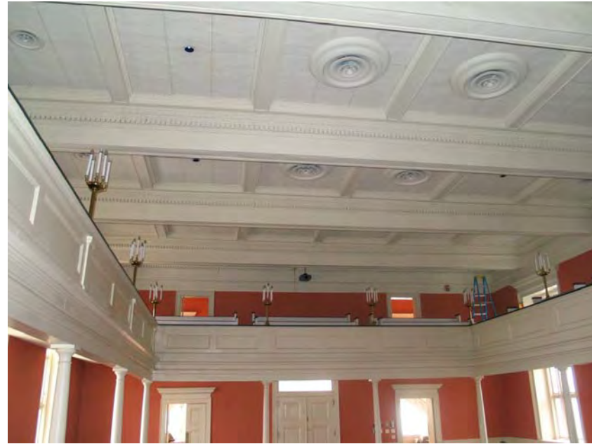
12 Ceiling Diffusers in Sanctuary
