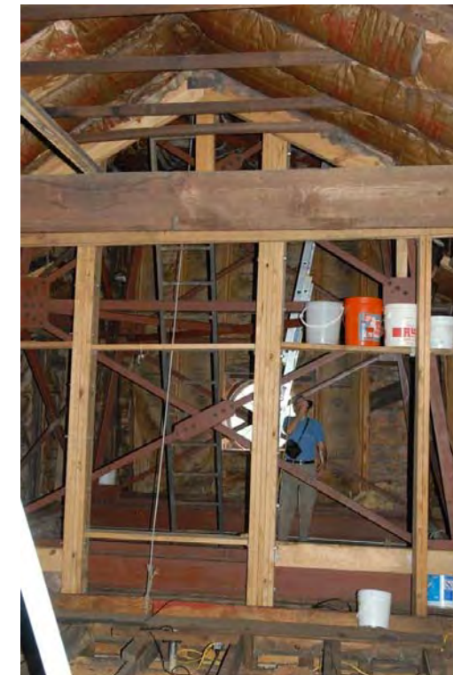
Buckets are lined up for drip water collection (time frame unknown)
